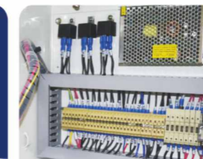
Terminal box inside
